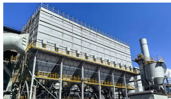
Baghouse dust collector
